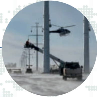
CANADA 130 km 240 kV transmission project
